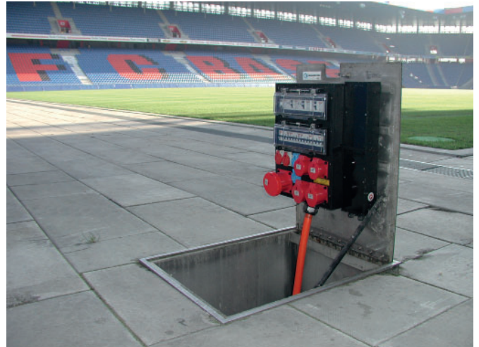
Underfloor distributor system, St.Jakob-Park stadium in Basel
