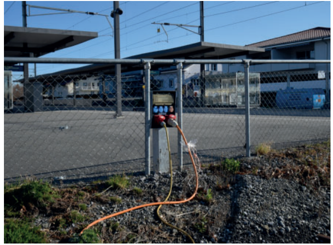
Power distribution box at Oberriet railway station
