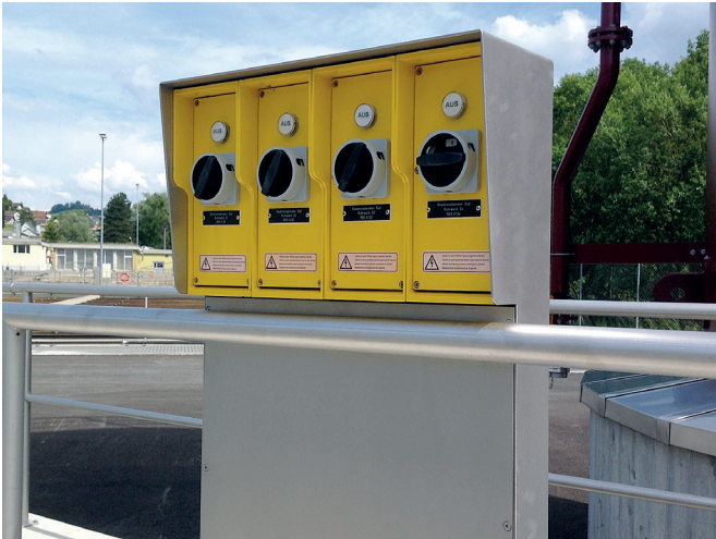
On-site switches, type 2812 yellow, sewage treatment plant Herisau
