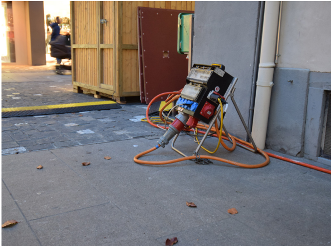
Mobile power distribution box in use at a market
