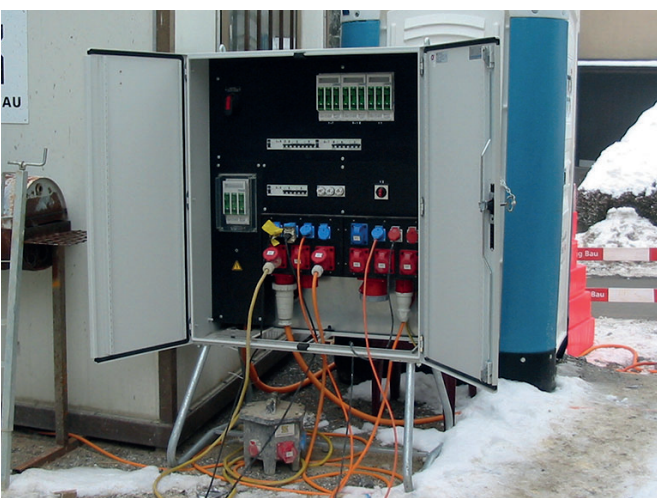
Main distributor on a construction site
