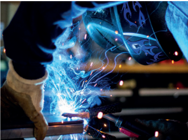
Ground clamp for the welding workstation
